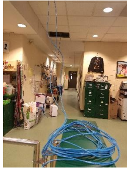
Extensive New Wiring
